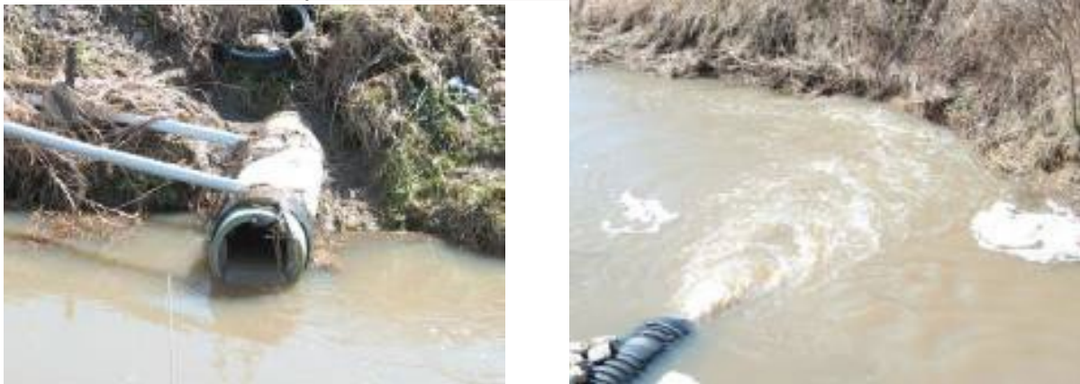
Figure 3: Two pipe outlets where frequent periods of submergence occur.
