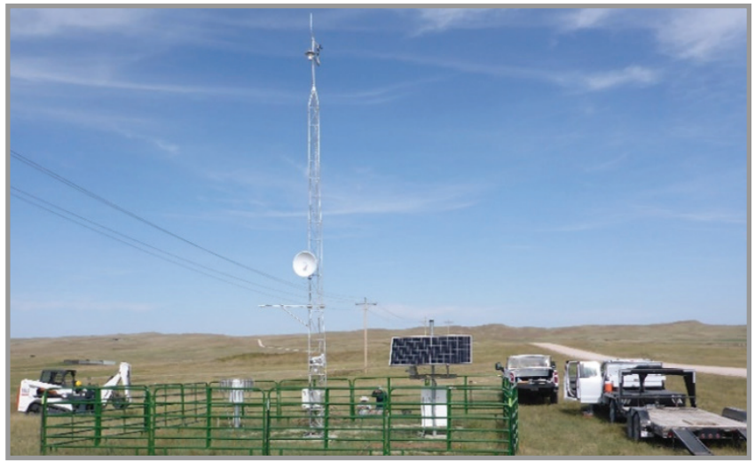
Figure 25.—A Upper Missouri River Watershed Project (Mesonet) site in Crook County, Wyoming.
