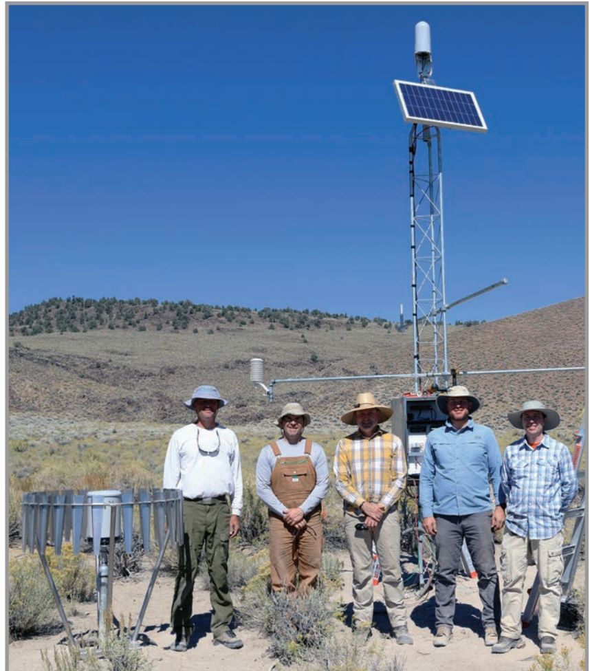
Figure 18.—As part of an agreement with the Bureau of Land Management, a crew installed three new Soil Climate Analysis Network sites near Mono Lake, California.
