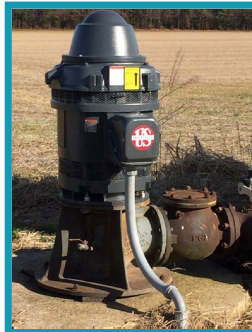
Irrigation Systems and Pumping Plants
