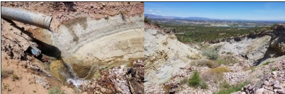
Figure 2-2: Coyote Canal Erosion
