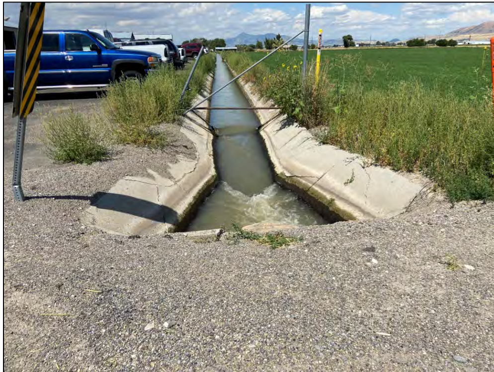
Photo 14: Looking north at a concrete lined ditch within the Central Canal Company Area.
