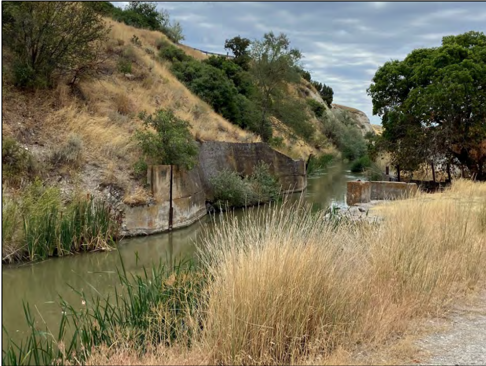
Photo 5: Lined portion of the Hammond Canal near the dam in the canyon area, looking southeast.
