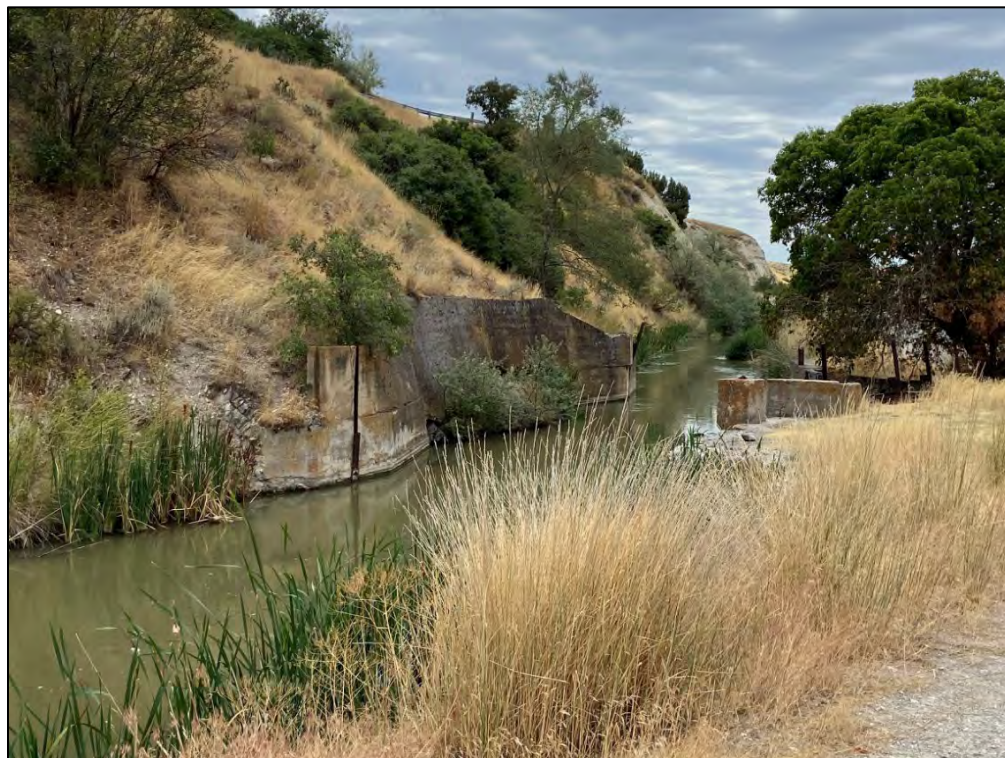
Photo 6: Lined portion of the Hammond Canal near the dam in the canyon area, looking southeast.
