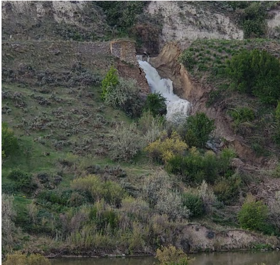
Figure 2.1.1.2. 2020 Hammond canal breach.
