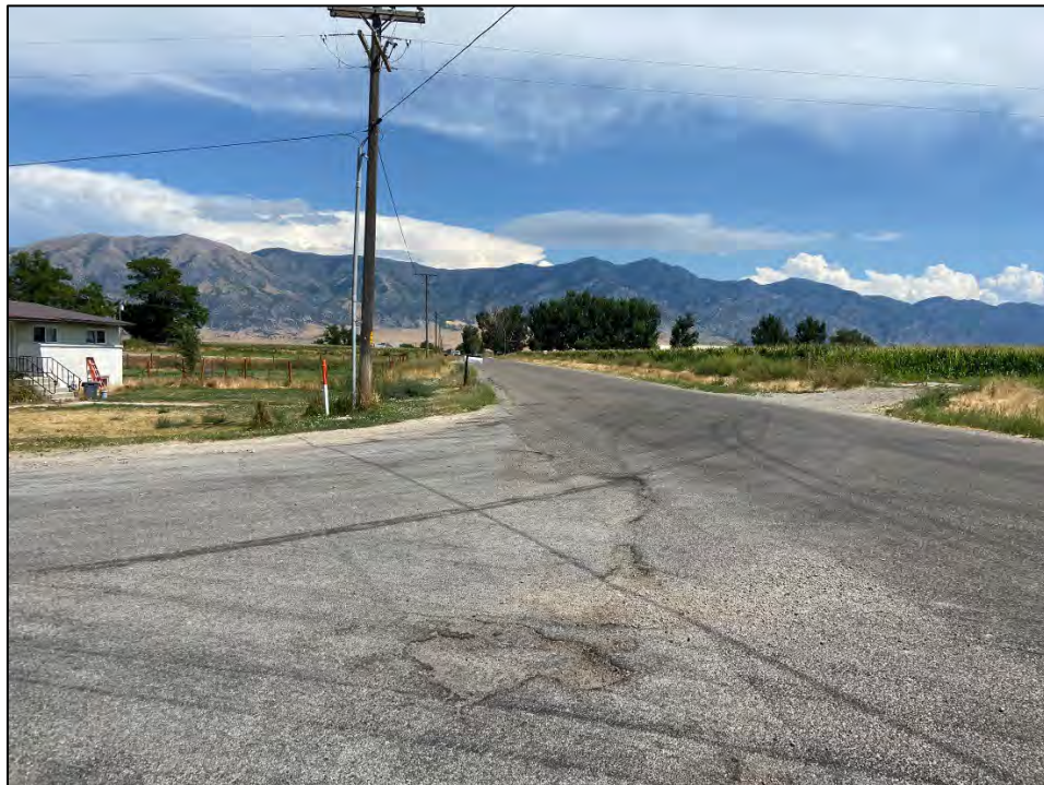
Photo 12: Location in Bear River City where proposed pressure irrigation improvements would occur, looking east.
