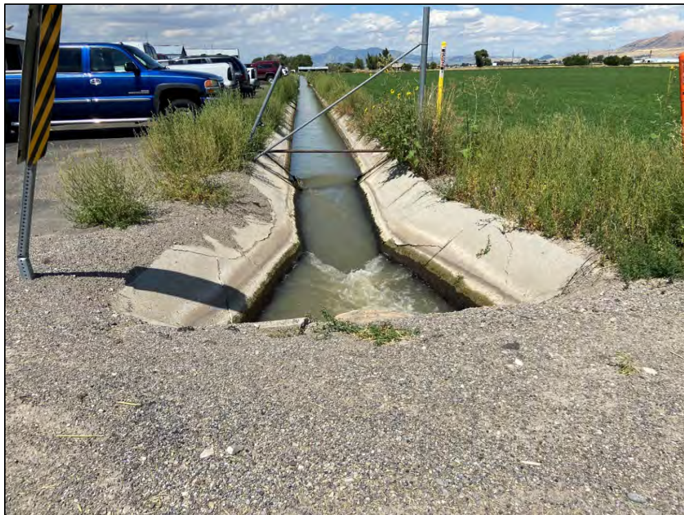
Photo 17: Looking north at a concrete lined ditch within the Central Canal Company Area.
