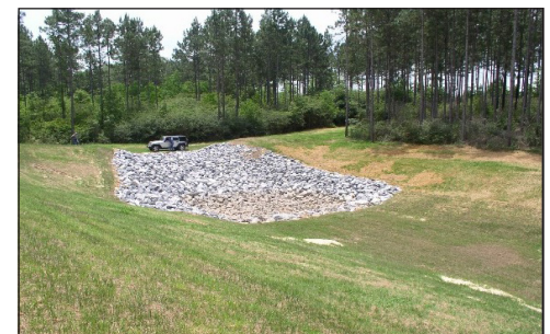
A combination of practices like grasses waterway and grade stabilization is a tool that can be incorporated into your conservation plan.
